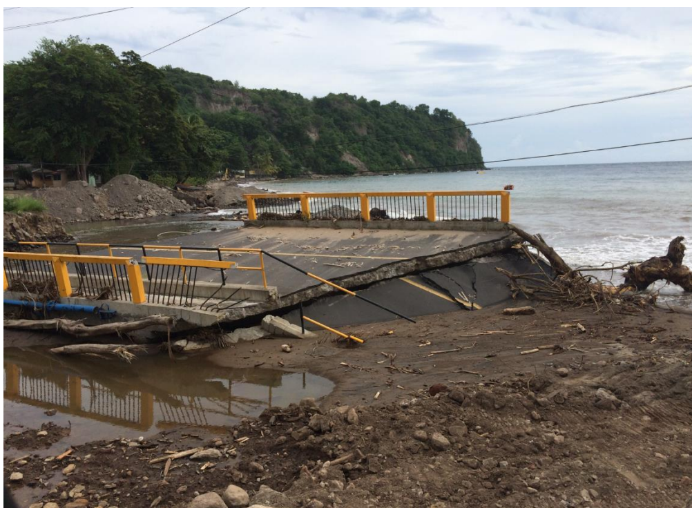
Dominica: bridge destroyed by Tropical Storm Erika, August 2015.
